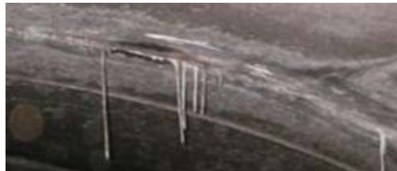
Figure 2: Moderate cracking and efflorescence on the underside of the liner [1].
