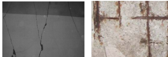
Figure 1: Crack observed in the lining of Longxi tunnel (left) [5] and concrete spalling with exposed reinforcing steel. (right) [1].
