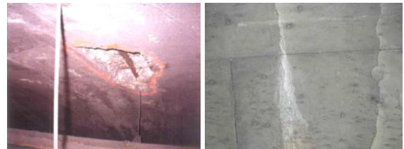
Figure 2. Examples of spalling (left) and crack with efflorescence (right) [5]
